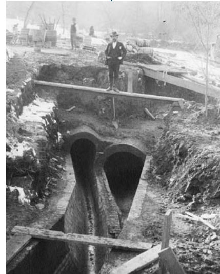
Building sewer overflows at 14th Street and Piney Branch, NW, December 8, 1893.
