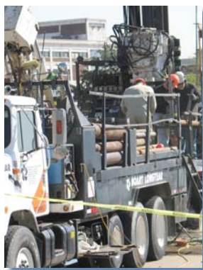
Truck-mounted drilling rigs take soil borings in the District to determine the CSO tunnel alignments.
