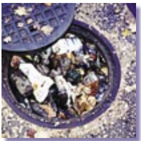
A trash-clogged combined sewer system can cause sewer backups and local flooding.
