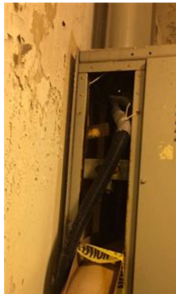
Water intrusion through the electrical service line
