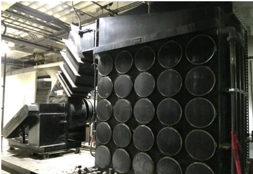
Odor Control Cannisters
