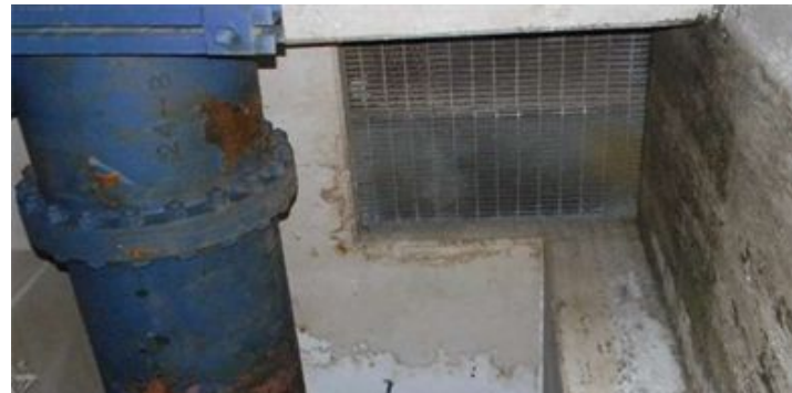
Water intrusion from equipment hatch
