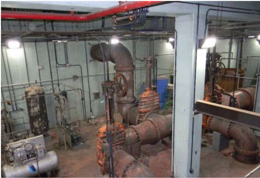
Inoperable valves on sanitary discharge piping
