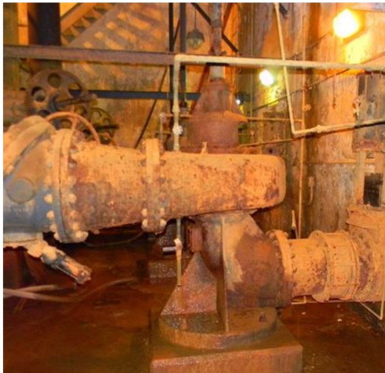
Leaking Stormwater Pumps
