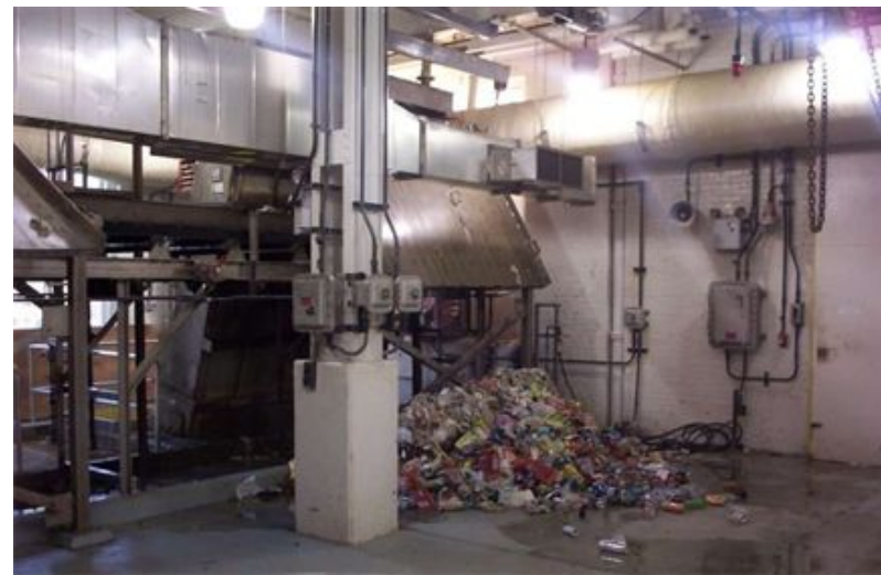
Lack of conveyance, washing and compacting
