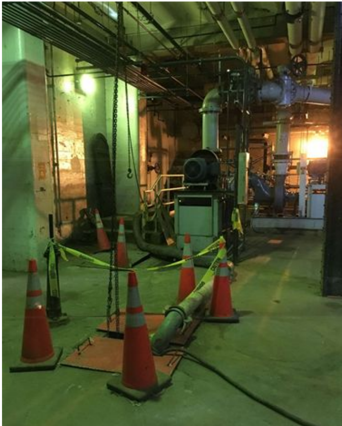
7 Low area pumps
