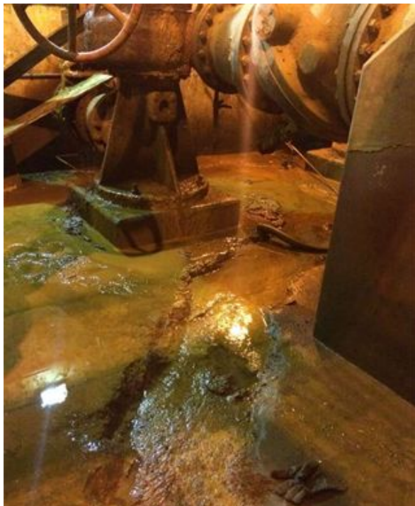
Valve leaking in dry well
