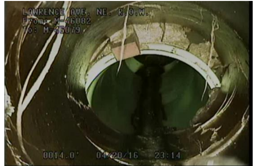
Montana Ave 18" VCP, deformed, blocked
