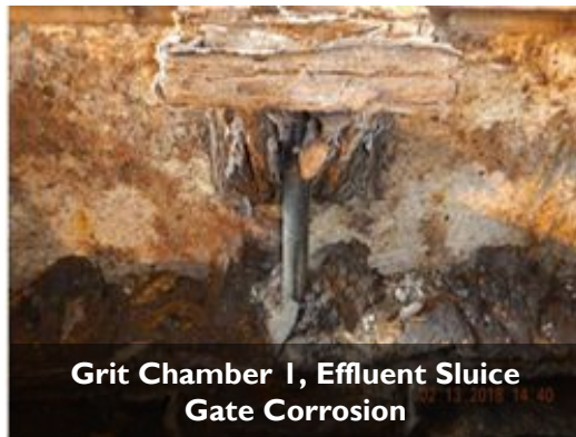
Grit Chamber Building I Concrete Corrosion
