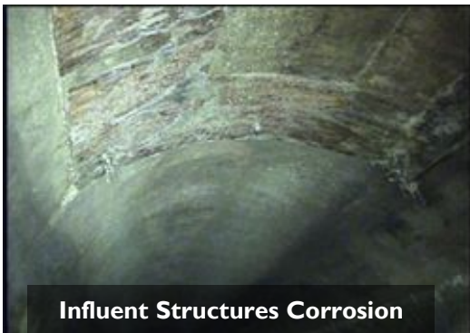
Grit Chamber I, Effluent Sluice Gate Corrosion
