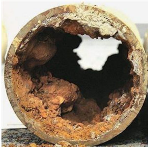
SDWM unlined Cast Iron pipe tuberculation
