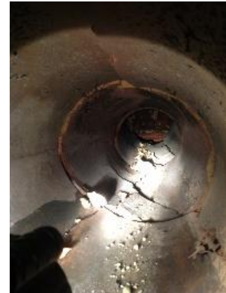
Vitrified Clay Pipe collapsed Small Dia. sewer
