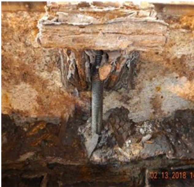
Grit Chamber Effluent Sluice Gate
