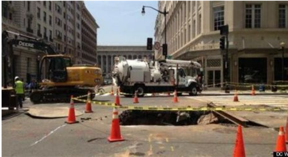
Sewer sinkhole, 14th Street blocked between New York and Pennsylvania Avenues NW
