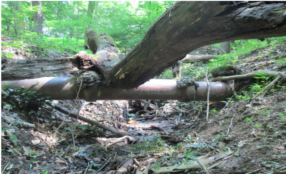
10" VCP Sewer pipe, installed in 1914, near Morrow Dr NW, located in Rock Creek Park.
