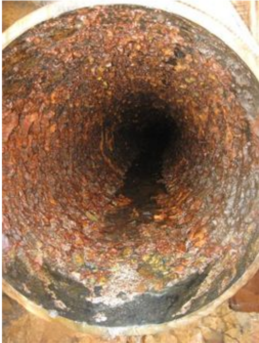
30-inch Tuberculated cast iron pipe (Rhode Island Ave)
