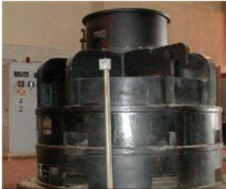
RWWPS I 1930s Original Motor
