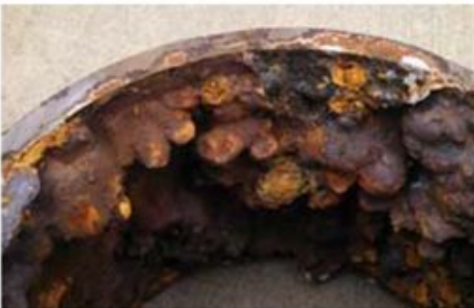
Pipe break, 8-inch tuberculated cast iron pipe Colonial Village
