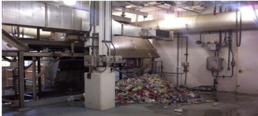
Lack of conveyance, washing and compacting
