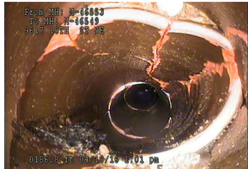
10 th St at Otis St, NE (10" VCP, deformed, broken)
