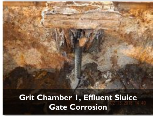
Grit Chamber Building 1 Concrete Corrosion
