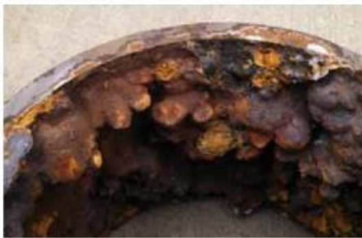
Pipe break, 8-inch tuberculated cast iron pipe Colonial Village
