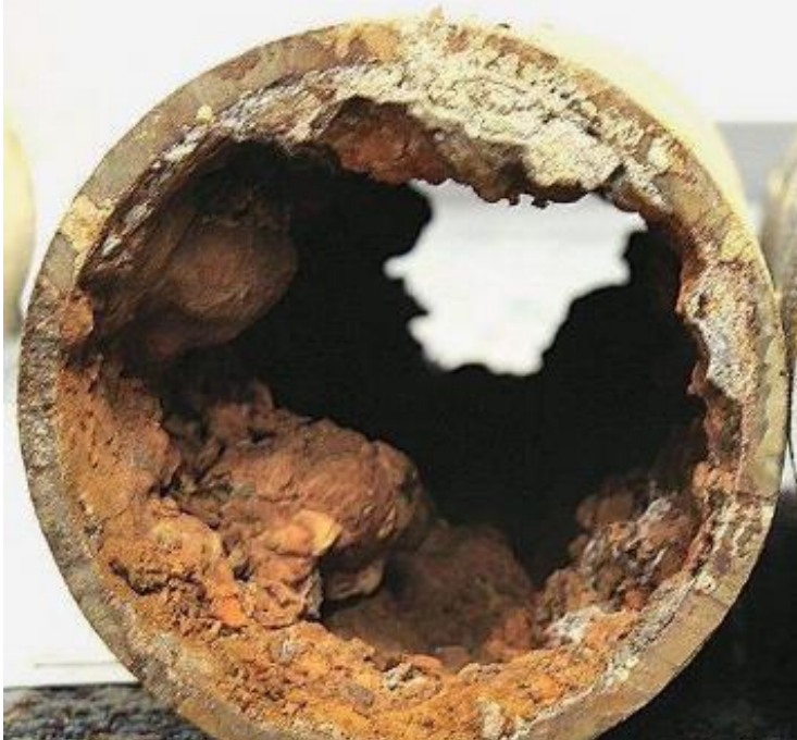
Small Diameter Water Main unlined Cast Iron pipe tuberculation
