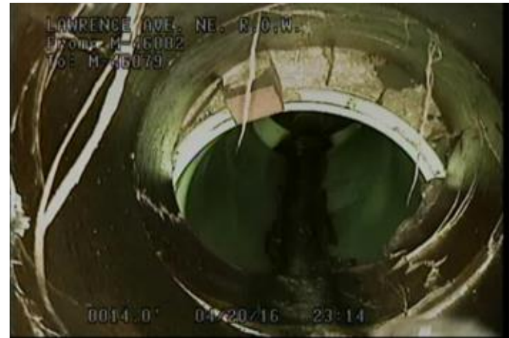
Montana Ave 18" VCP, deformed, blocked
