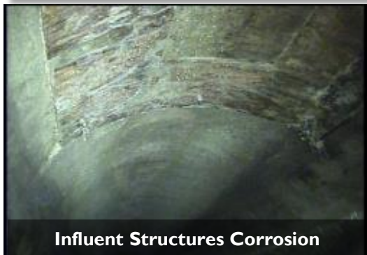
Grit Chamber 1, Effluent Sluice Gate Corrosion
