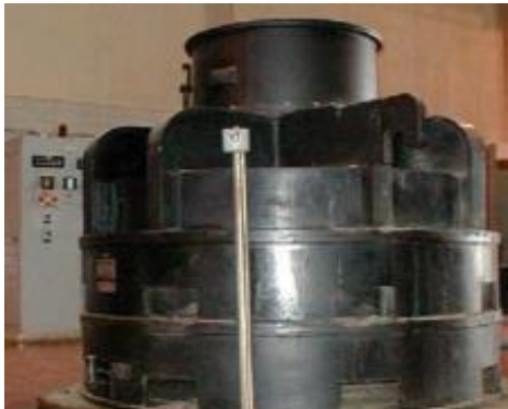
RWWPS 1 1930s Original Motor
