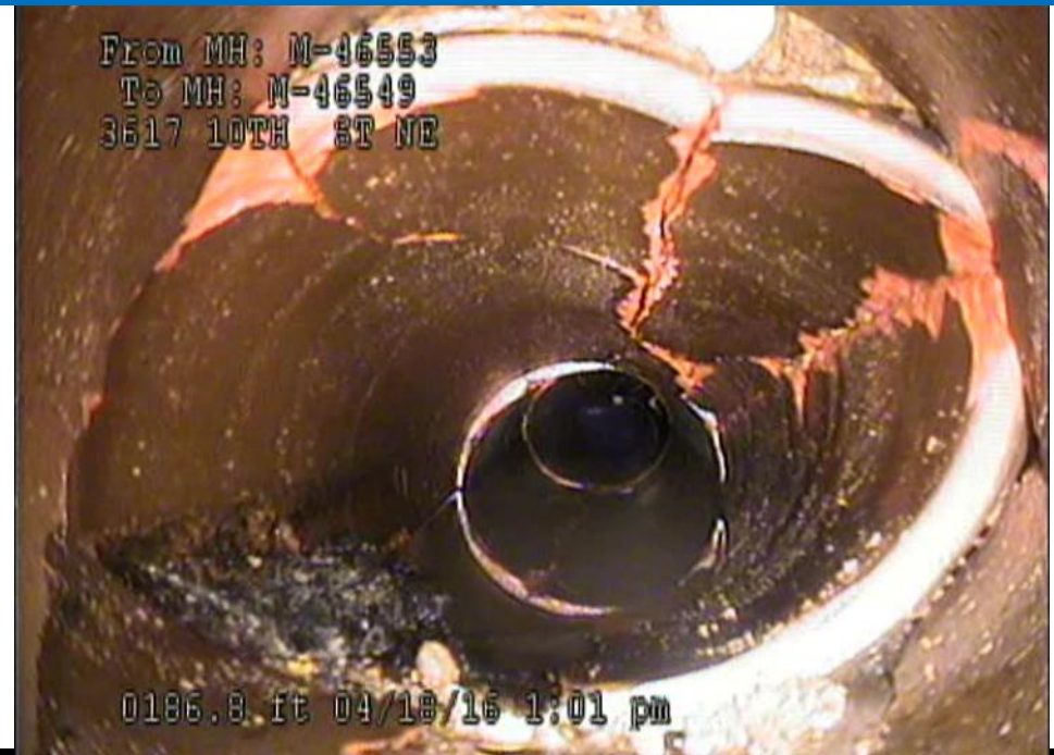
10th St at Otis St, NE (10" VCP, deformed, broken)
