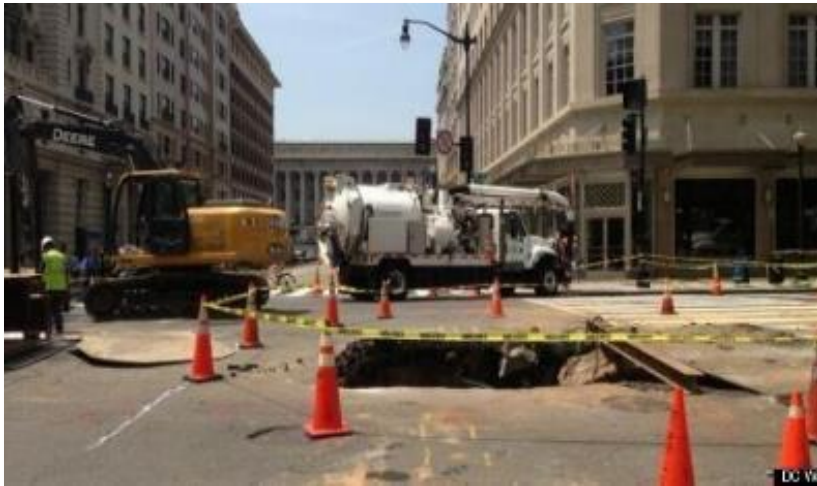
Sewer sinkhole ,14th Street blocked between New York and Pennsylvania Avenues NW
