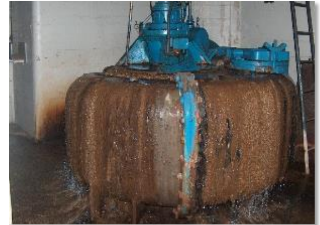
Failed Stormwater Pumps
