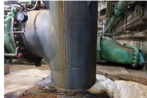
PSW Pump - Seal Failures
