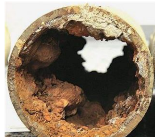
SDWM unlined Cast Iron pipe
