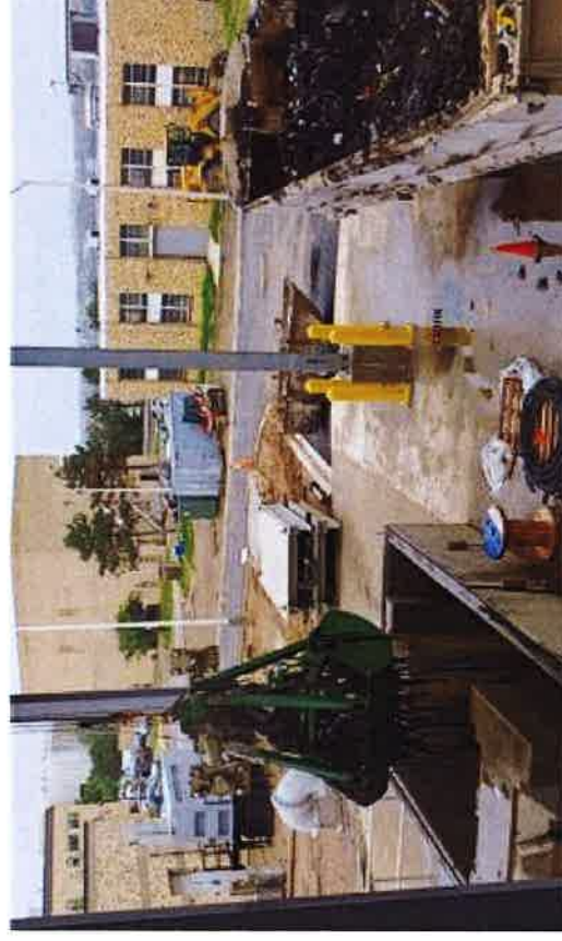
Trash, Debris and Solids Removal from Screening Shaft at Tunnel Dewatering Pumping Station
