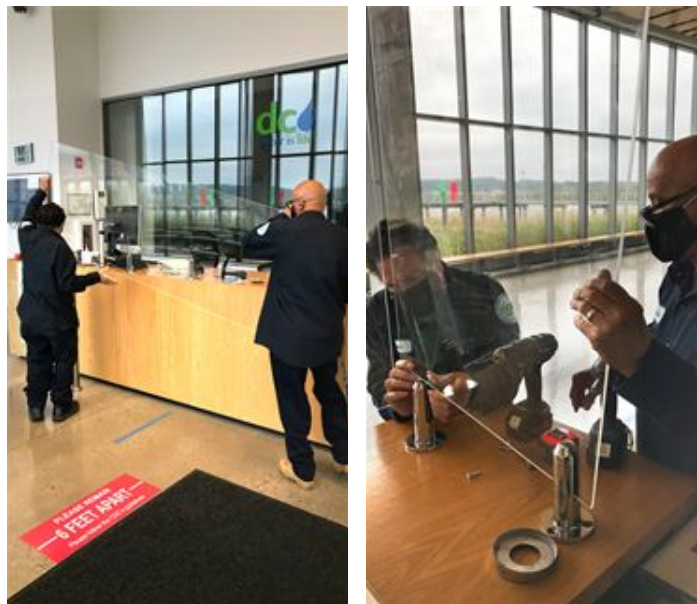
Carpenters Robert Stewart and Coy Jeffries installed custom Plex-Shield at the HQO Security Desk
