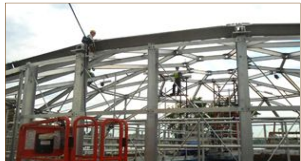
Gravity thickener upgrades
