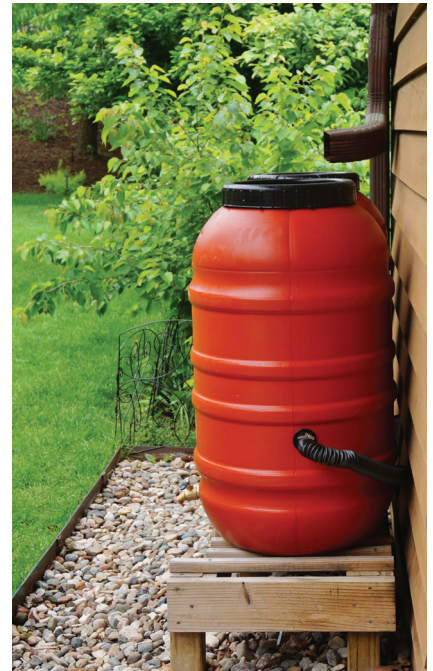
Rain barrels capture and store rain water for uses around the home and garden. Contact DOEE's RiverSmart program: doee.dc.gov/riversmart
