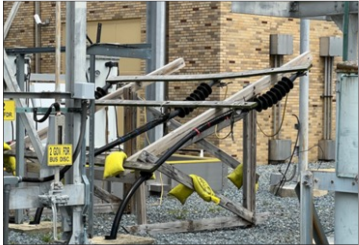
Two new power cables ready to be connected at the PEPCO Main Substation at Blue Plains
