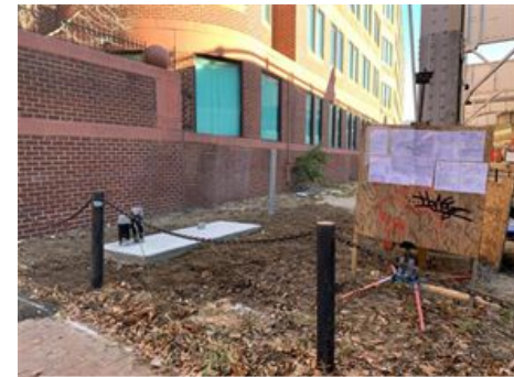
Electrical Pad at CSO-024
