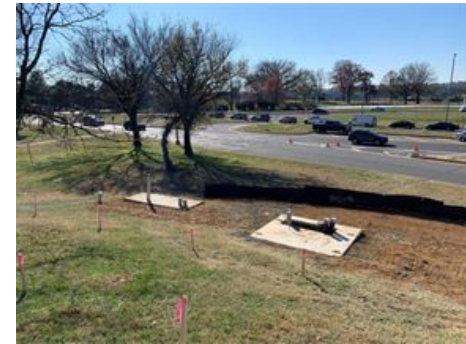
Electrical Pad at CSO-020
