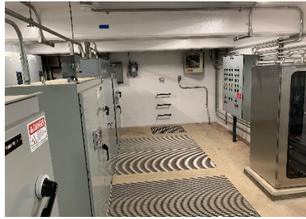
Stormwater Overflow Control Room
