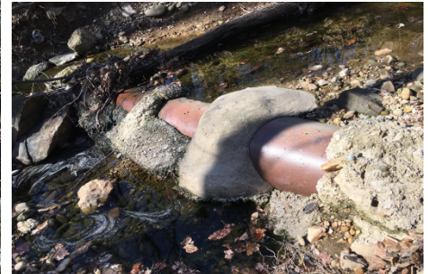
Sewer Rehab (Pinehurst exposed sewer)
