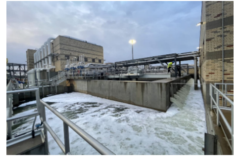
Blue Plains Clarification at Wet Weather Treatment Facility
