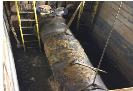
30 Inch Water Main
