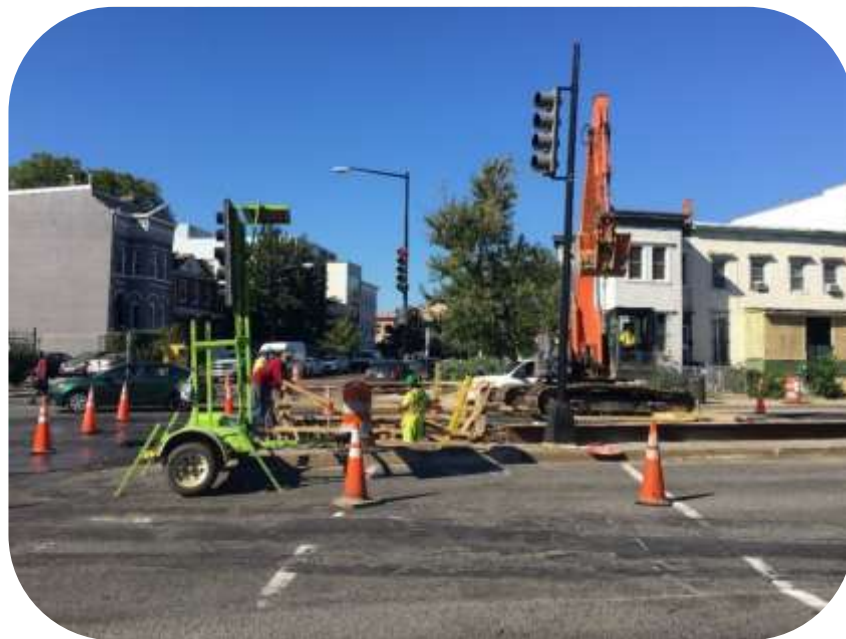
Figure 1: Working on 48-inch low pressure water main at R and 6th Streets NW.
