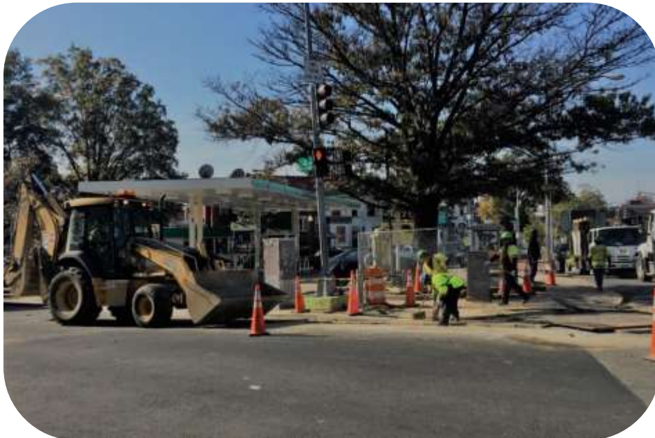
Figure 2: Restoring curb and sidewalk on 3 rd Street and Rhode Island Avenue NW.
