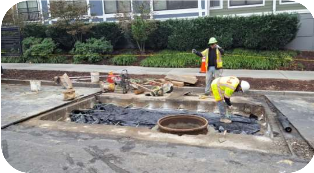
Figure 6: PEPCO manhole on Rhode Island Avenue NE near 8th Place NE.
