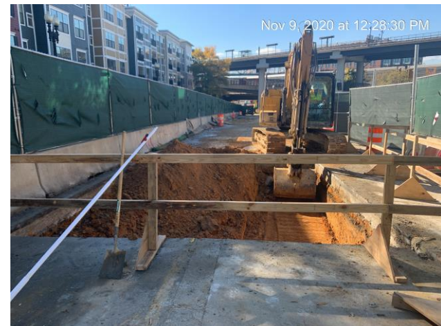
Excavating the muck pit for jet grout work in the Rhode Island Avenue NE median area
