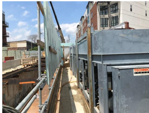
Soil freeze system behind noise barriers
