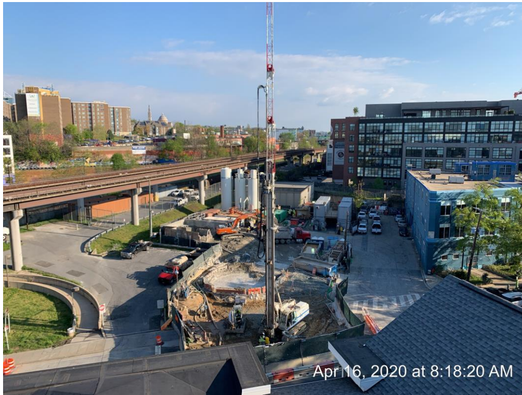
View of the jet grout rig working on ground improvement for the adit
