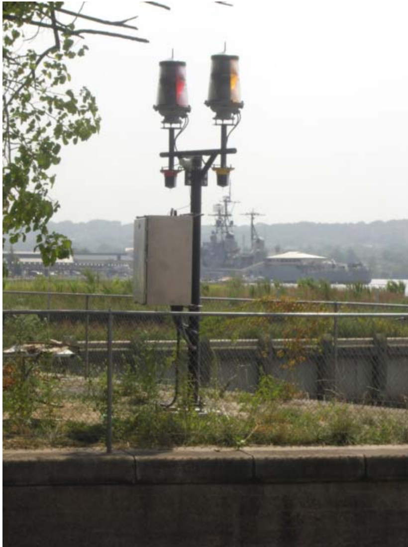
Figure 11: CSO Warning Lights on Anacostia River
